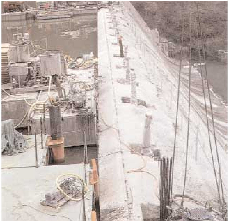
Mountainous terrain required that all of the work be done from barges tied to the upstream face of the dam.
