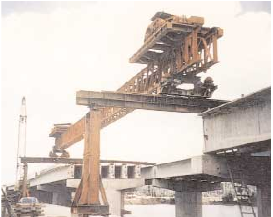
Modified T-beams replace the originally designed I-beams.
