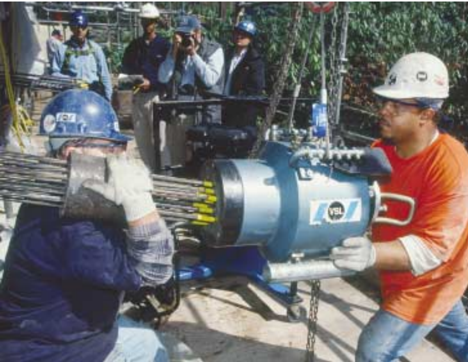
Fig. 6: Multi-strand tendons were carefully stressed in stages using a hydraulic ram. Here, technicians position extender nosing (left) and ram over the strand tails in preparation for stressing
