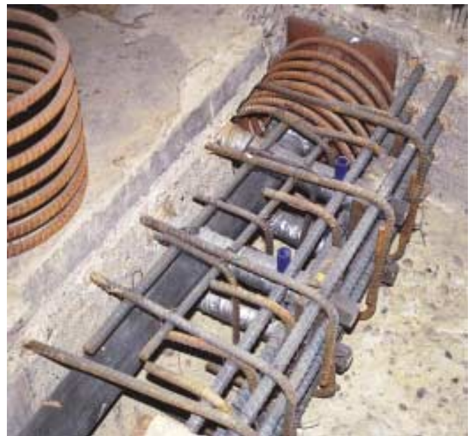
Fig. 5: View of a typical multistrand stressing end anchorage for one of the three primary cantilever girders spanning in the north-south direction
