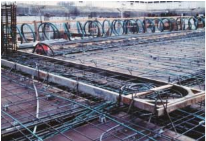
Job site at the Entry Pavilion, Community Hospital of the Monterey Peninsula
