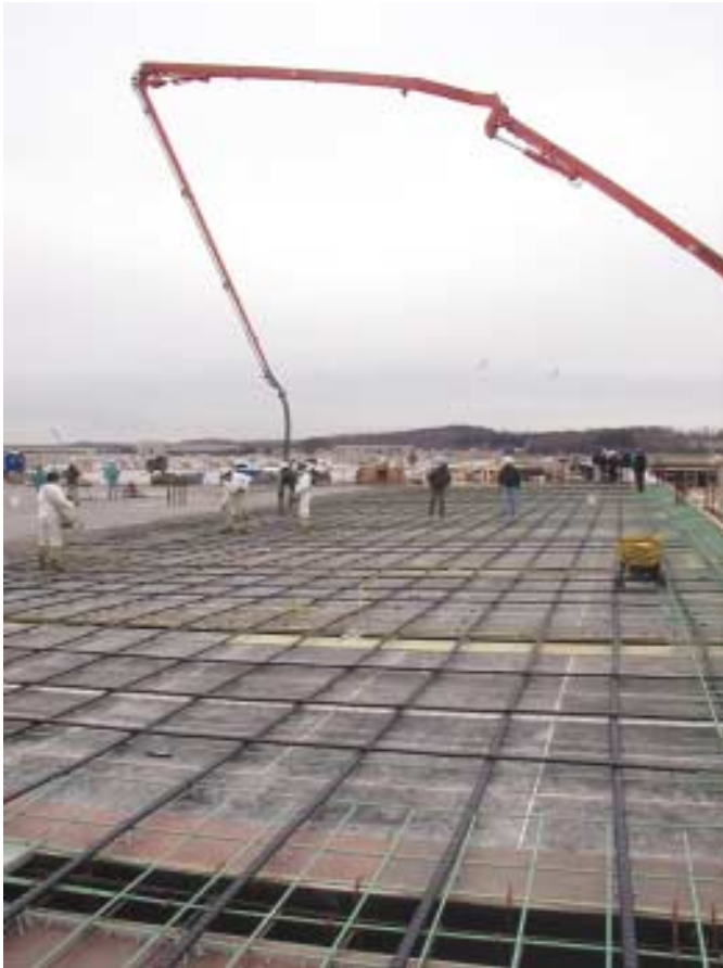
Fig. 1: The elevated deck of the new parking structure at BWI airport is constructed as a post-tensioned concrete beam and slab system
