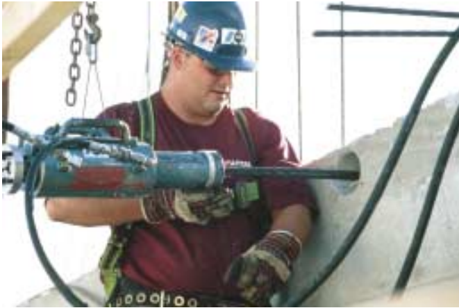
Fig. 5: The post-tensioning contractor used a special two-strand hydraulic ram to stress the tendons in the slab at the new BWI airport parking structure
